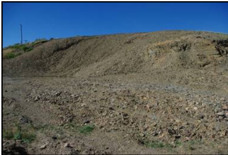
Figure 79: Current impact at borrow pit 151_BP02
