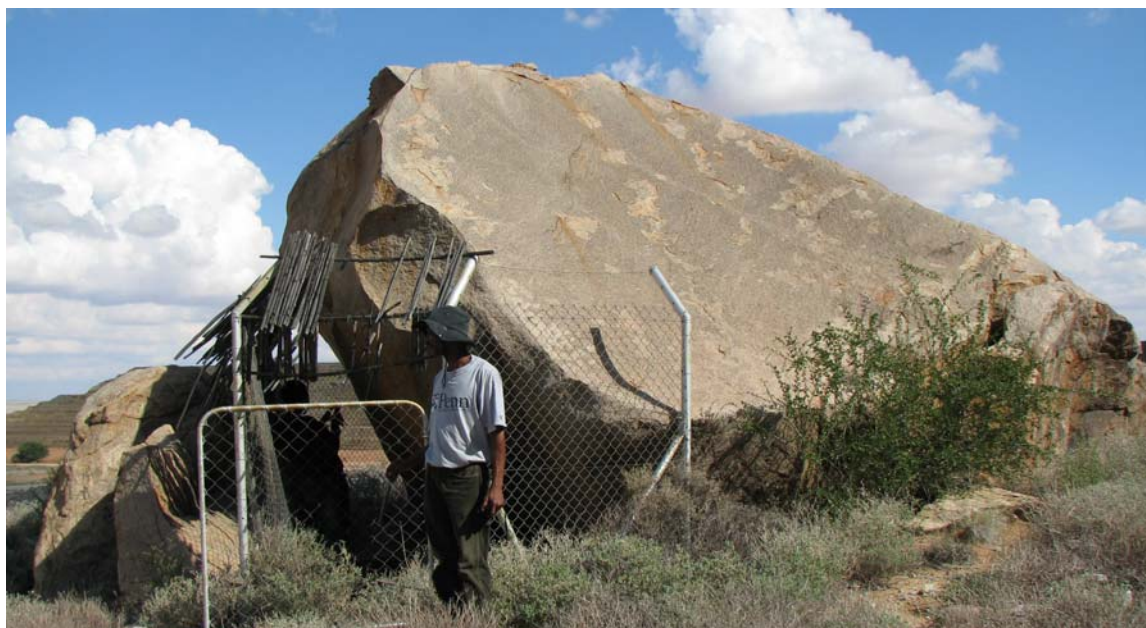
Painted boulder with protective fence and reed roof (needs repairing).
