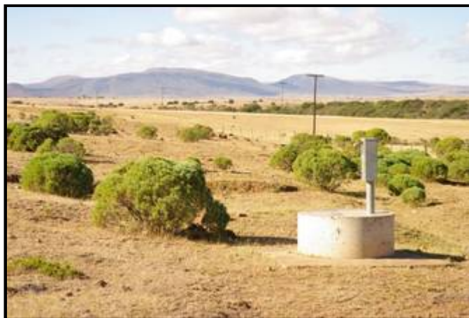
Figure 11: Existing water infrastructure, with fenced fields in the background
