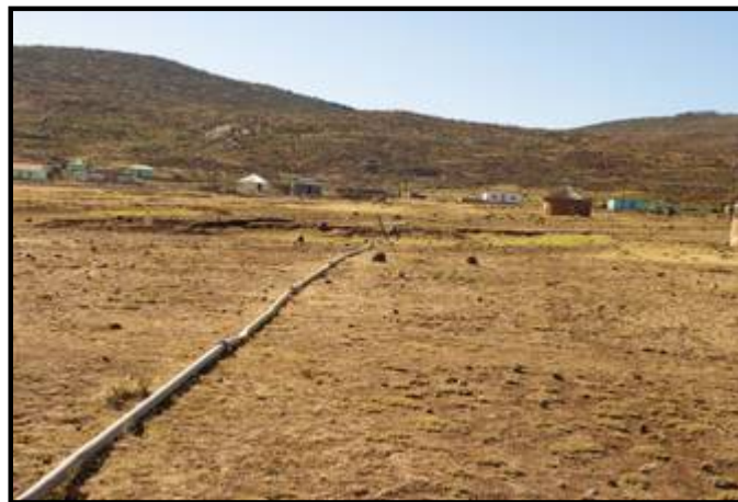
Figure 48: Existing water infrastructure at the western part of Tshatshu Village
