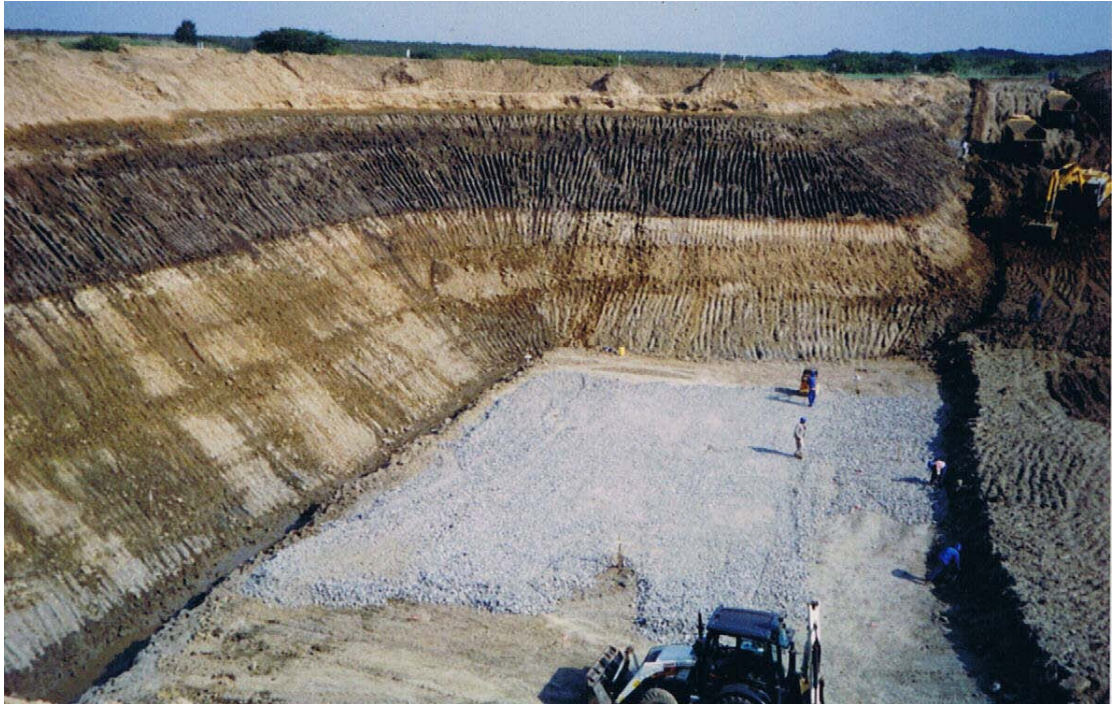
Cretaceous layer being covered in crushed stone to stabilize floor for construction of caissons, 2 August 2005.
