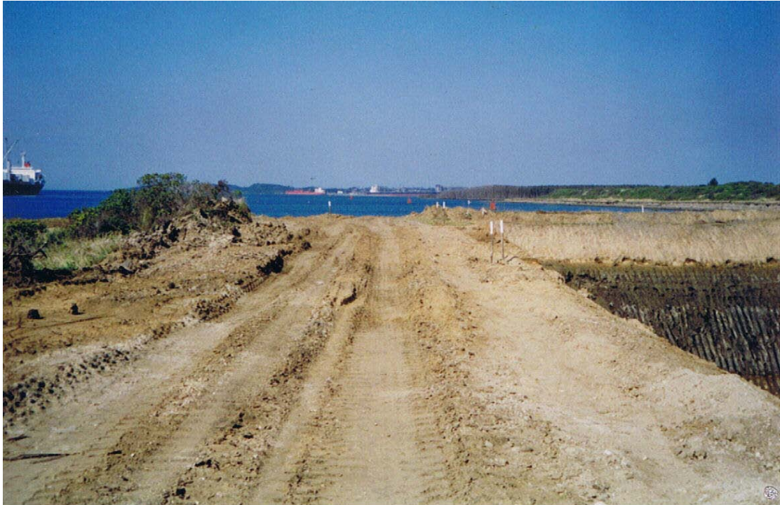
“Wall” constructed between harbour and dry pit excavations on eastern side of harbour.
