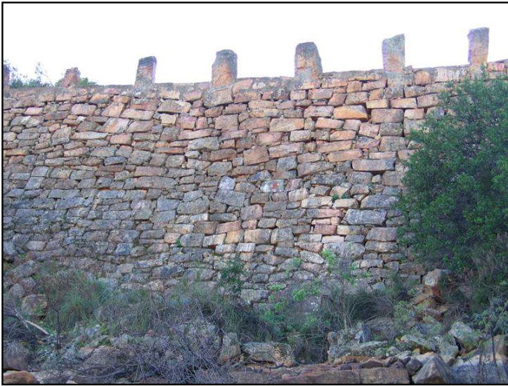
Plate 30: CDE14. At this point a large retaining wall had to be built to support the 1930's road as it traversed a steep section of the valley.
