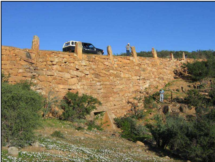
Plate 31: CDE31. Another section of the 1930 road built up with a retaining wall. This section crosses a small river valley and had to have a concrete culvert inserted at its base. Such culverts were very commonly employed along the length of the road.
