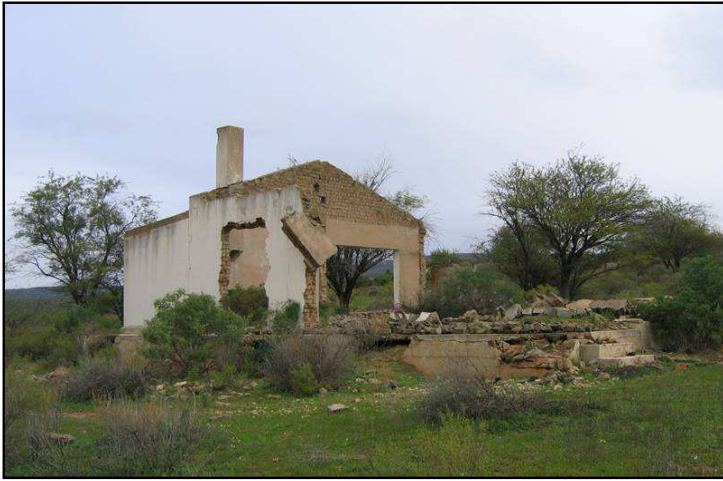
Plate 25: CDW44. An example of a modern house that is already in ruin. This house has an inscribed date of 1944 on a drain indicating that it is older than 60 years and hence is protected.
