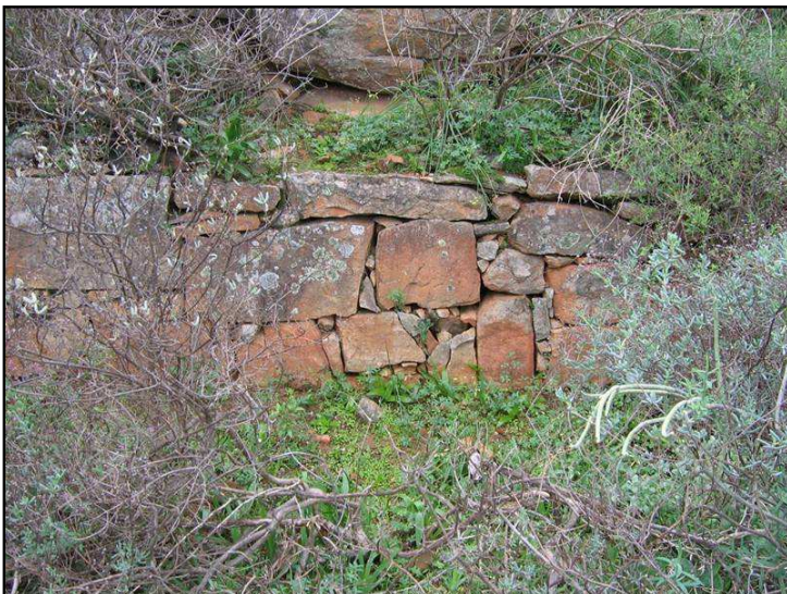
Plate 27: CDE08. This small retaining wall is located on the upslope side of the 1860 road and serves to hold up a small sandy embankment above the road.
