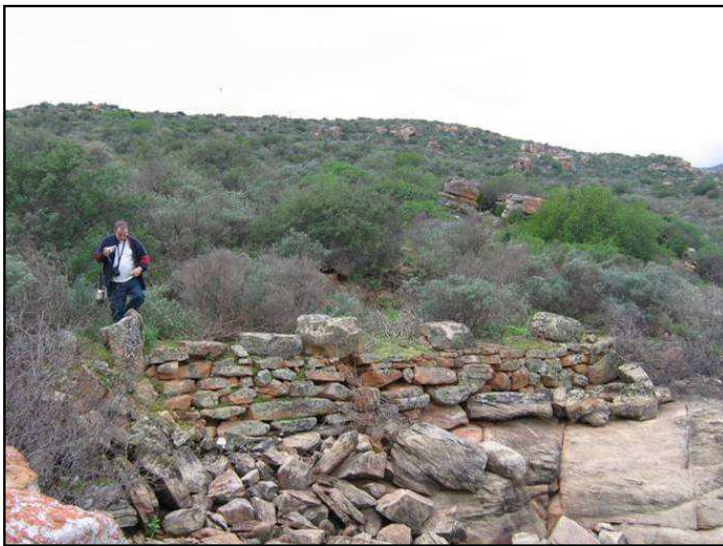
Plate 26: CDE08. This section of dry stone retaining wall on the 1860 road is located immediately alongside the current full supply level. It supports the road from beneath.
