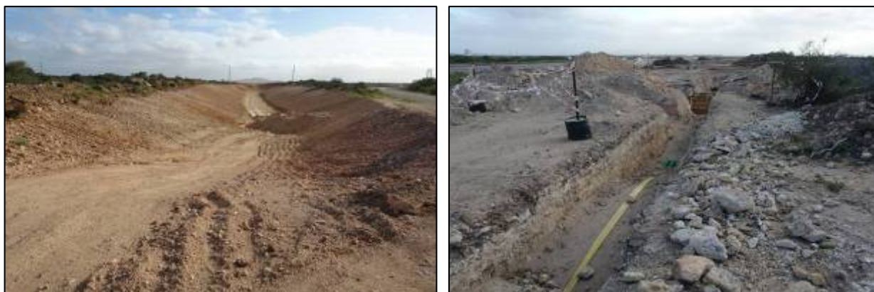
Figs 33-34. Road building in the western part and pipe line construction along the N2 national road in Zone 6.
