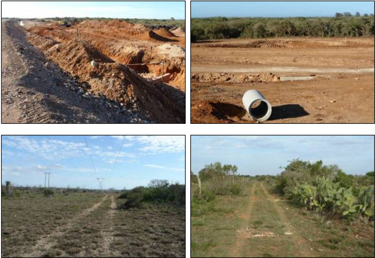
Figs 99-102. Different views of road and pipe line construction along the western side of zone 11 and small scale disturbances by power line and farming activities.
