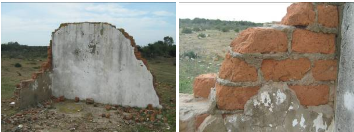
Figs 13-14. Remains of a possibly historical farmhouse (left) and a close-up of the bricks (right).
