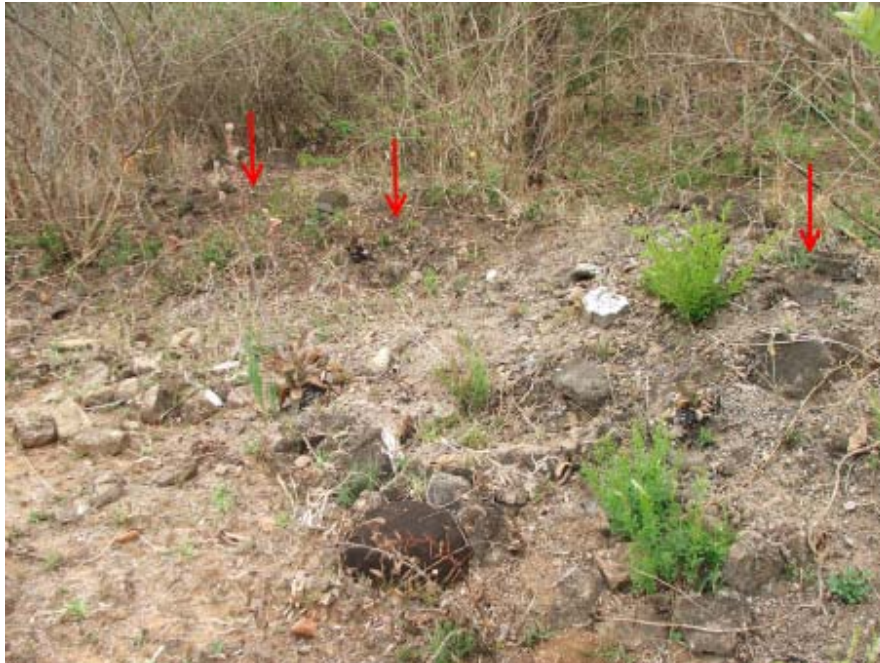
Fig. 5. Site 4. Site HD 4. The arrows indicate rubble and the foundations of walls.
