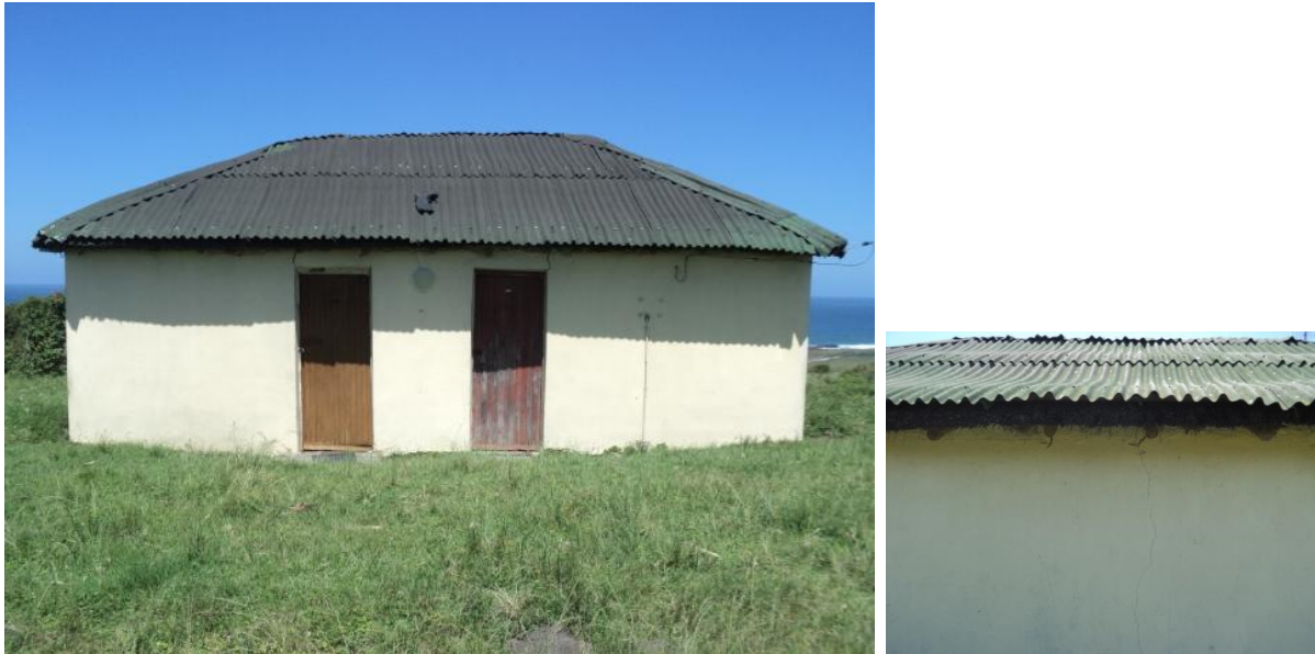
Figure 4: View of another house that will be demolished to make way for the proposed staff accommodation units. On the right is a close view of the roof of the structure. These were thatched of wheaten-straw and later on when straw start to perish, aluminium sheeting was laid above as indicative on the right photo.
