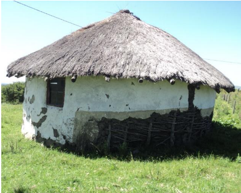
Figure 1: View of the roundavel structure that will be demolished. This, house is currently used by reserve employee.
