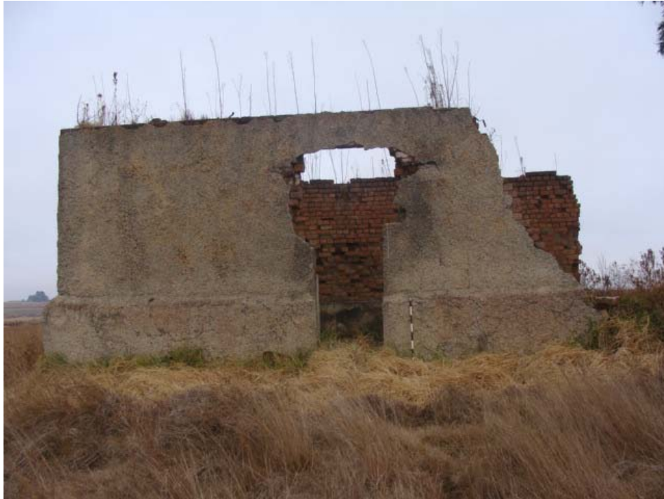
Figure 21 Front view of the ruin of the old church.
