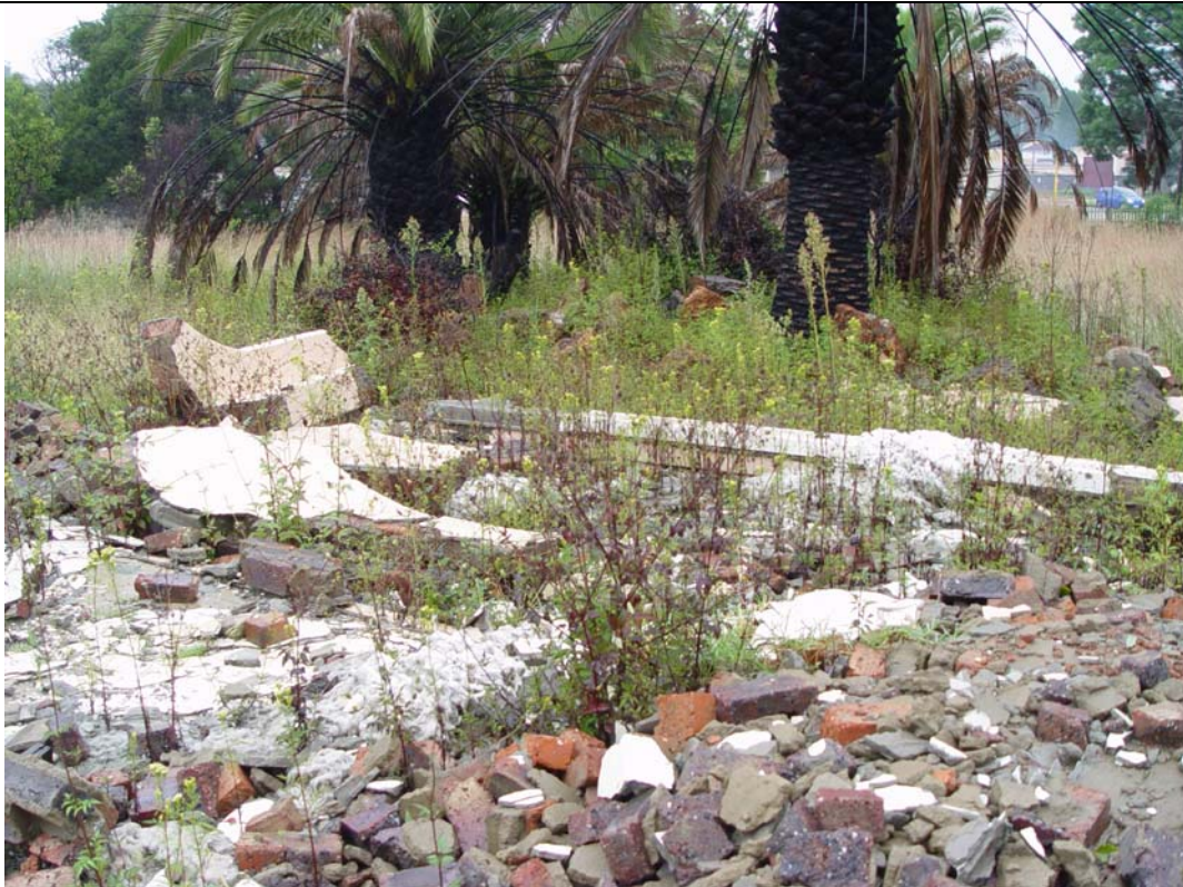
Figure 5: Remains of demolished house.
