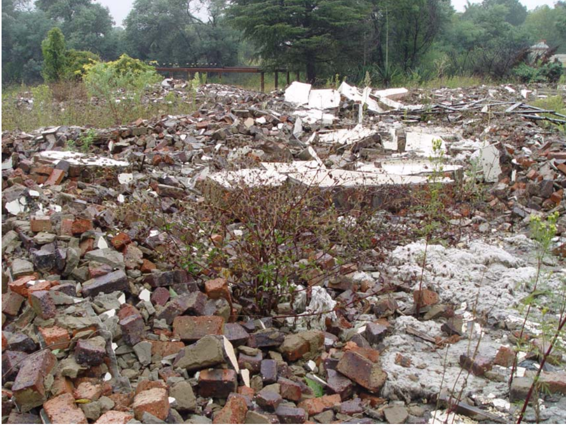
Figure 4: Remains of demolished house.
