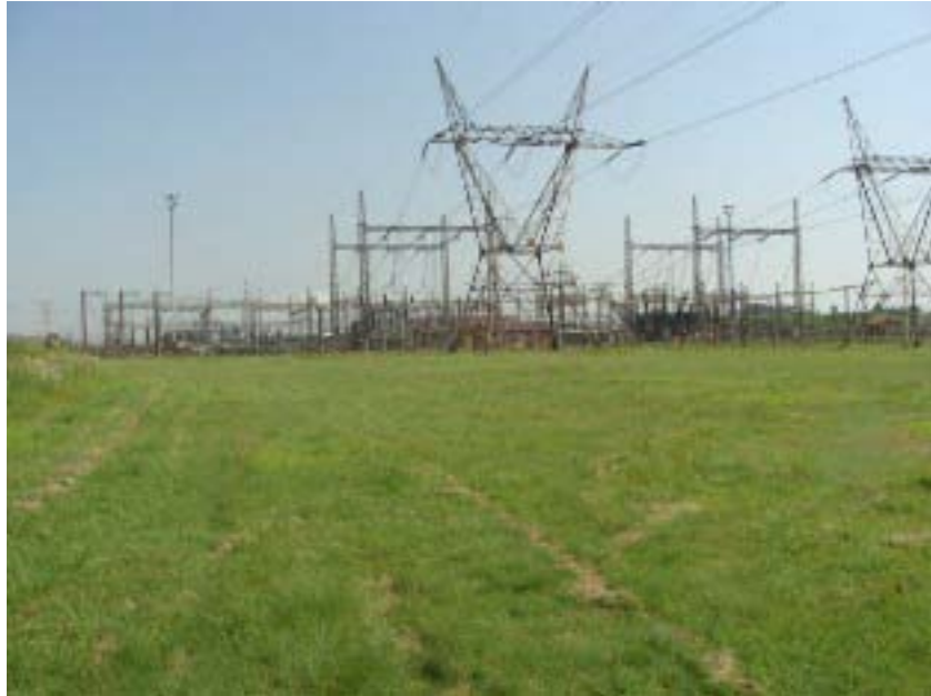
Figure 8: View of Kookfontein substation. The new line runs to the left of the picture
