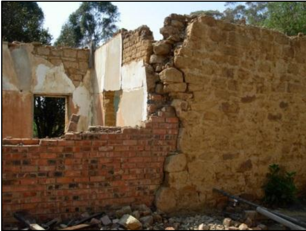
Figure 11 – Fired clay bricks indicating additions and reparation works
