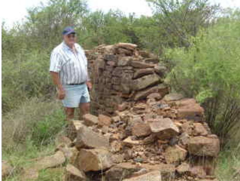
No. 1 Mr. Chris Smith next to one of the partially collapsed walls
