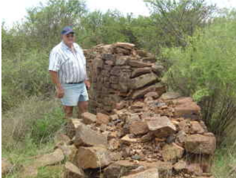
No. 1 Mr. Chris Smith next to one of the partially collapsed walls
