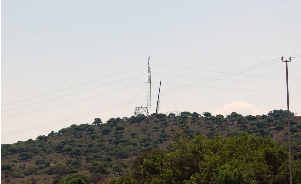
Plate 6-8: Construction of a high voltage power line pylon exposed against the skyline. View from photo site A24.
