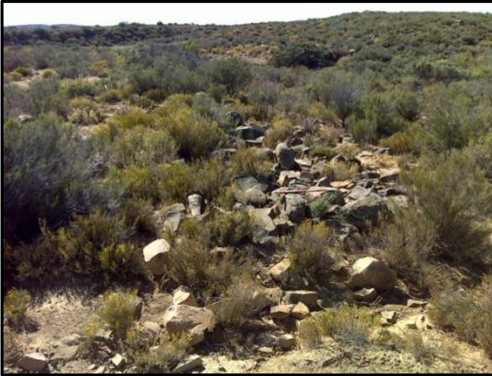
Figure 11. View of the collapsed portion of the dry packed stone wall adjacent to the farm gravel road (HVSTSW1).
