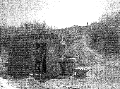
Photo 7: Scour valve at lowest point.
