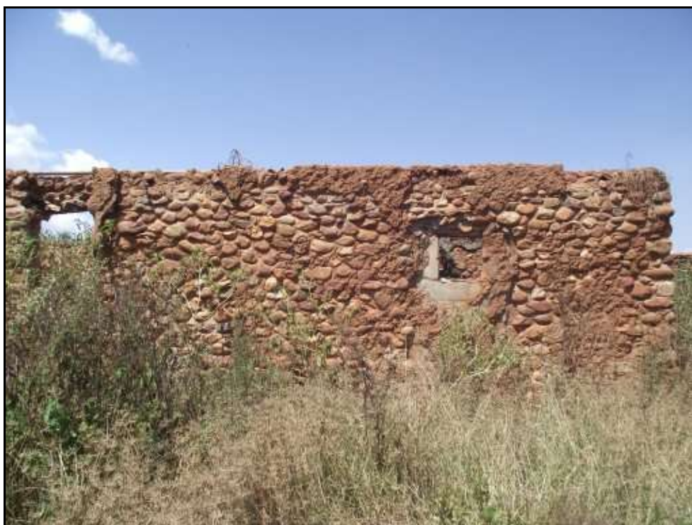
Fig. 33. Site CLB 23. Window frames of concrete, door frames of steel and stone and mortar lintels.
