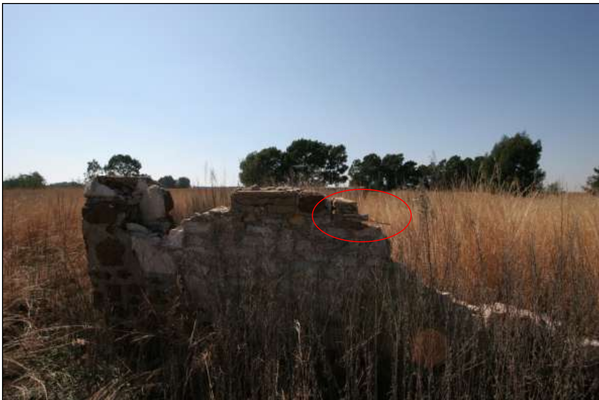
Figure 11: Detail of outer wall. Note the reinforced lintel (in red outline) as well as repairs to wall (different stone).
