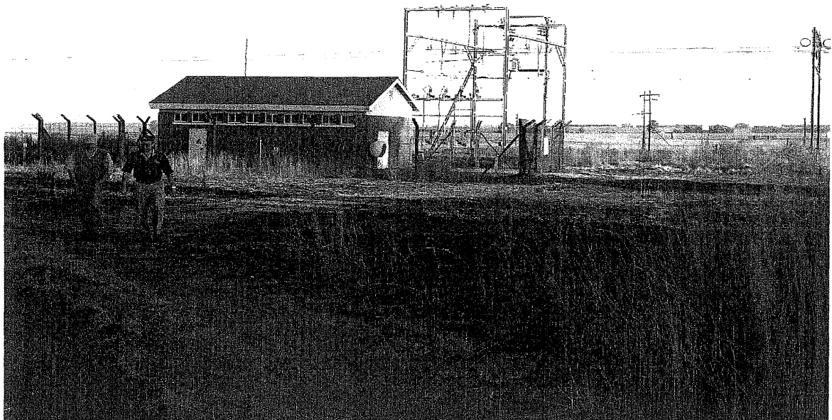
Photo 4. Existing Agent spoor net sub station (point of supply 2.)
