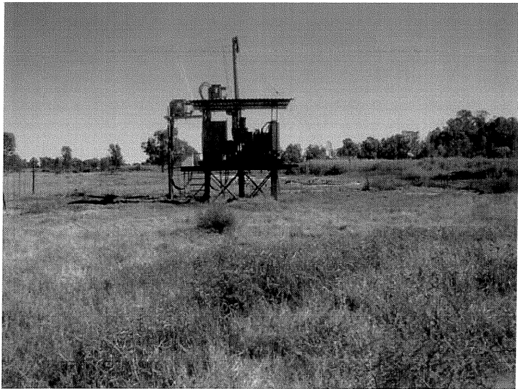
Figure 16. The pipeline section terminates at a pump house facility(above) and electrical substation (below) at the Vaal River (point H).
