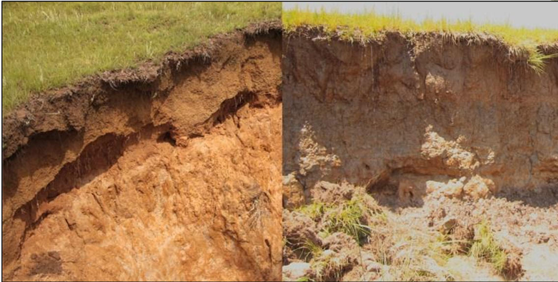
Figure 9: Erosion gullies at Sites A & C exposing geomorphological compositions of sub-surface deposits.
