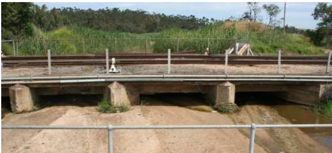
Figure 4. Silt accumulation under rail bridge on the Platteklip River near the confluence with the Diep River.
