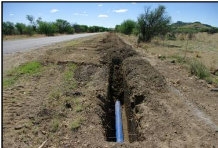
Figure 8: View of current development impact – Portions of the pipeline have already been closed up while open sections are visible in other places
