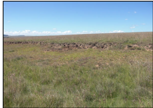
Figure 13: Erosion sections at the dam
