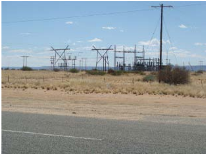
Figure 3: View of the ESKOM Substation close to the area.
