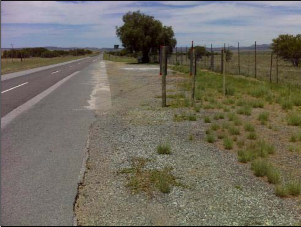
Figure 5. Example of other disturbances within the road reserve (picnic spots and sign boards).
