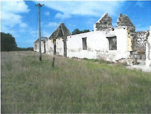
Figure 9. Rietfontein se Langhuis. Burnt out farm building
