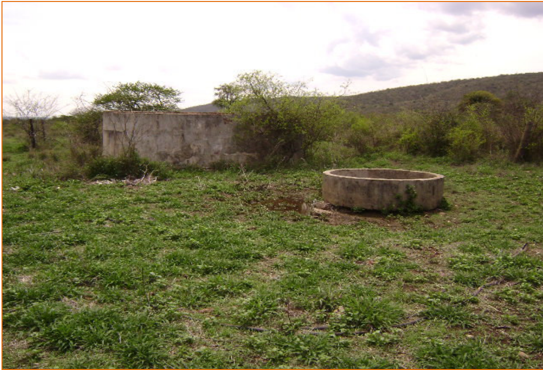
Figure 3: Some of the recent past infrastructure a concrete reservoir and livestock drinking trough.
