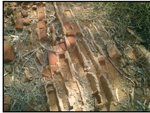
IMAGE 02: Collapsed clay brick wall at RP01 (Site RDP01)
