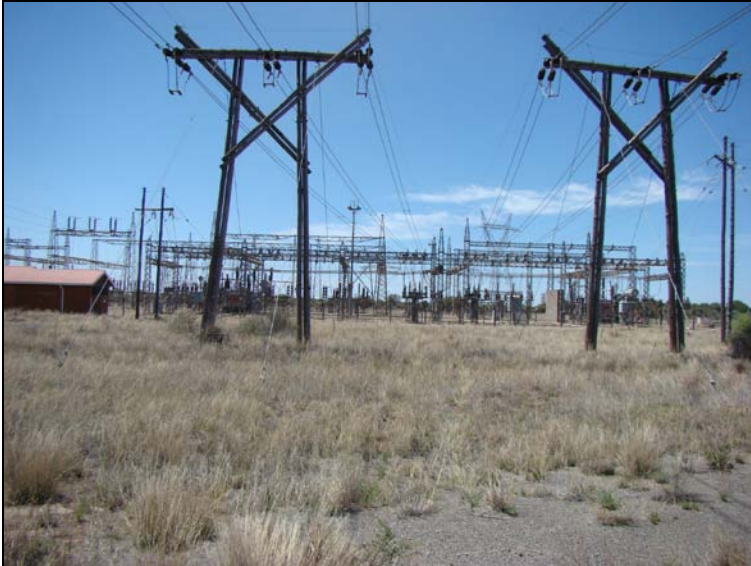
Fig.1 The Eskom sub-station at Lime Acres.
