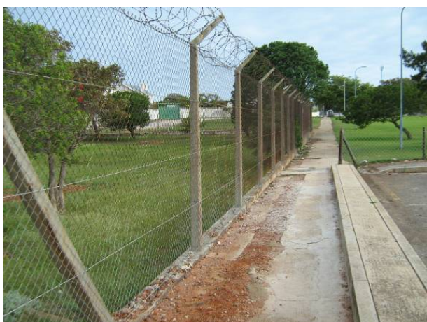
Fig. 7. View of the cement path and the fence separating the development (on the left) from Richmond Park (on the right). The two trial pits are visible within the fenced area.
