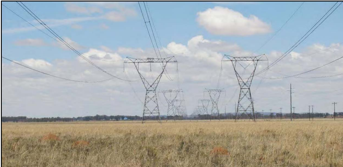
Plate 3: View of the transmission lines which run down the length of Dennehof farm, on the boundary with Jedwater.
