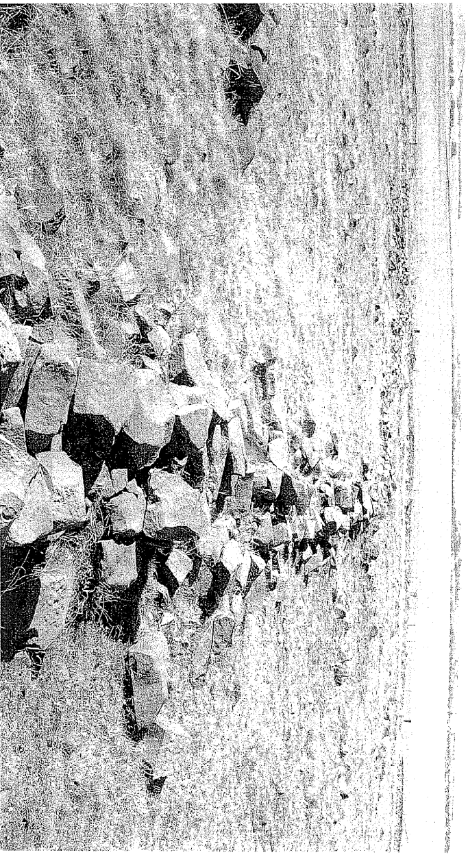
Photo 7. Dilapidated circular stone wall at LCL 001.
