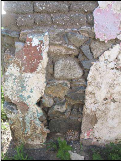
Figure 12: The point at which the cross-wall once met the front wall. Note stones to ~1 m only.
