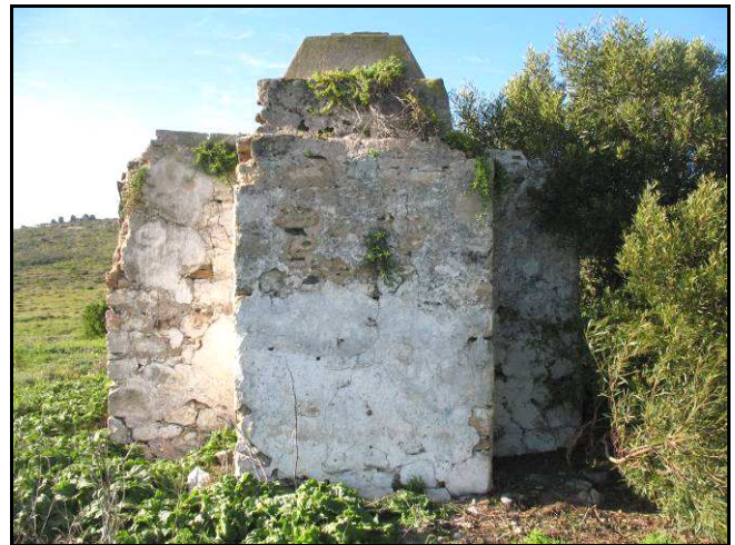
Figure 16: The hearth and chimney stack on the northern end of the building.
