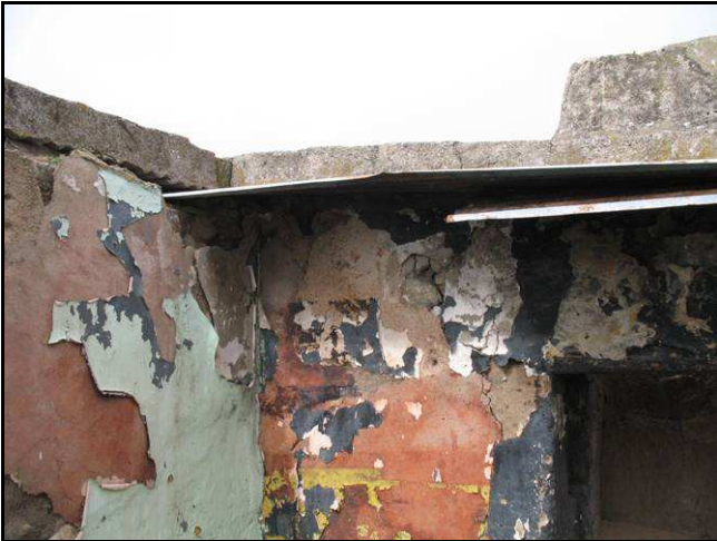
Figure 38: The remaining section of corrugated iron roof with modern bricks and cement above.
