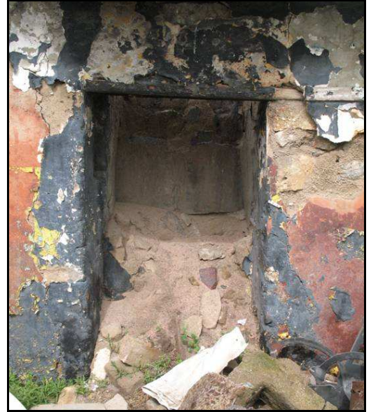
Figure 37: The inside of the hearth filled with rubble from the collapsed chimney.
