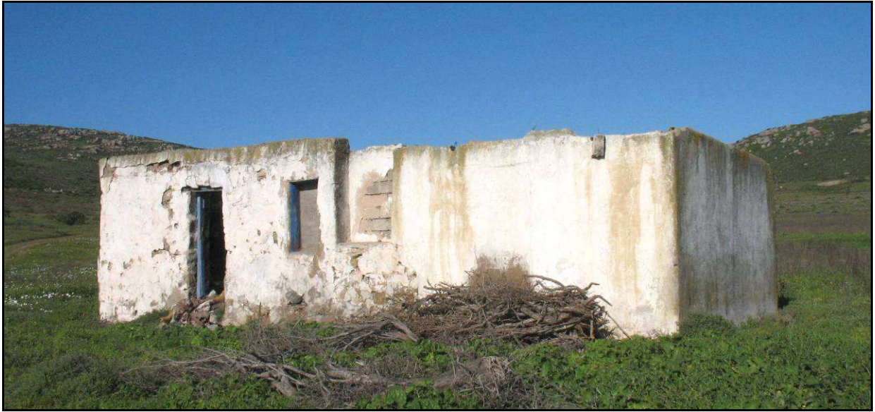
Figure 33: View of the front of SHB20-4 showing the differing walls of the original (left) and newer (right) parts.
