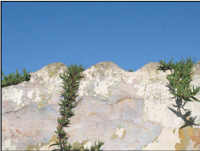
Figure 19: Detail of cement on top of the back wall showing the imprint of corrugated iron.
