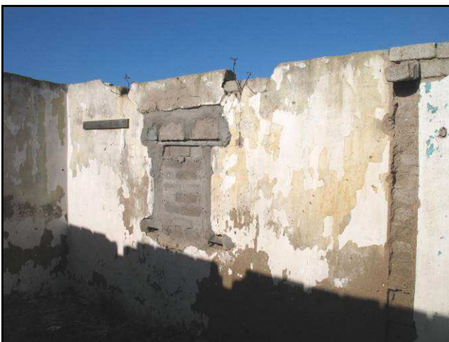
Figure 27: The bricked up southern window and the scar where the cross-wall used to be.
