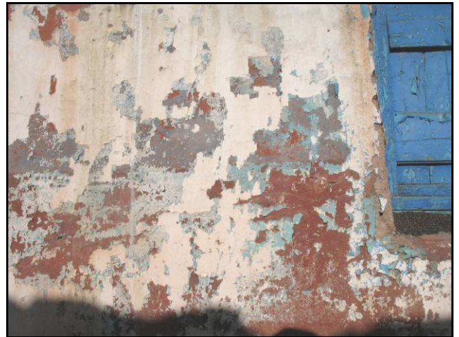
Figure 20: Detail of the interior paint. Part of the broken door is also visible.
