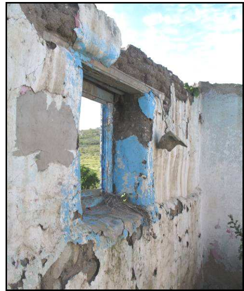
Figure 18: The wooden window frame and lintel in the back wall of the northern room.
