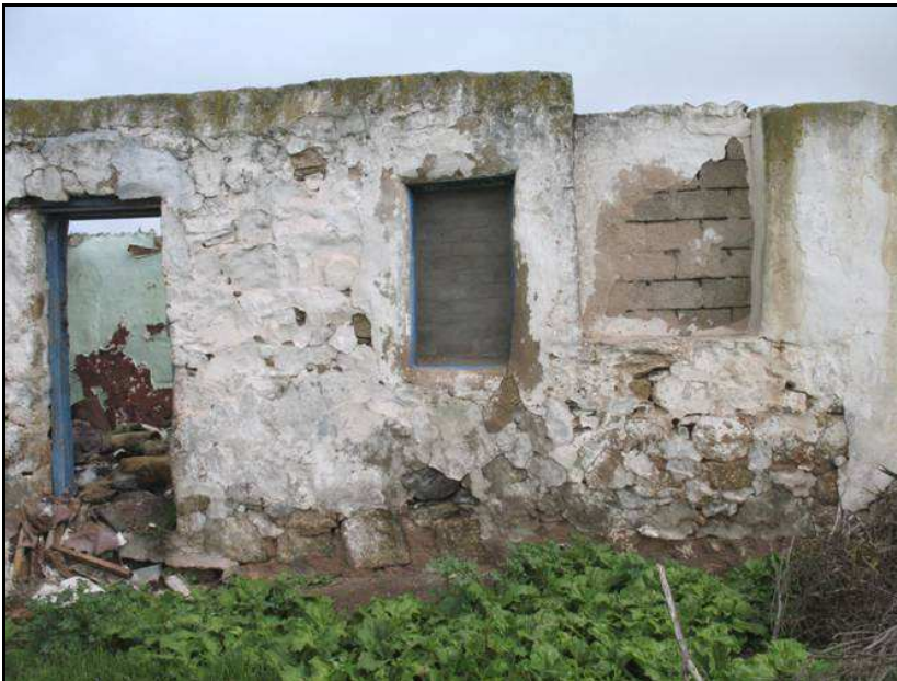
Figure 34: The central part of the front wall showing the peculiar bricked-up “window” alongside the other bricked-up front window.
