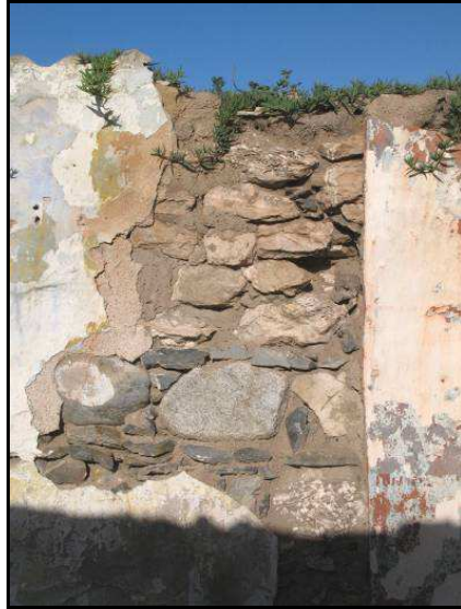
Figure 13: The point at which the cross-wall once met the back wall. Note stones to full height.
