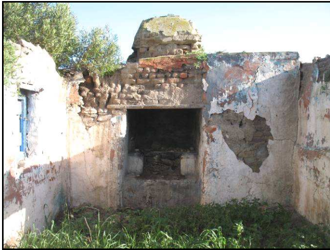
Figure 17: View of the hearth from the inside.
