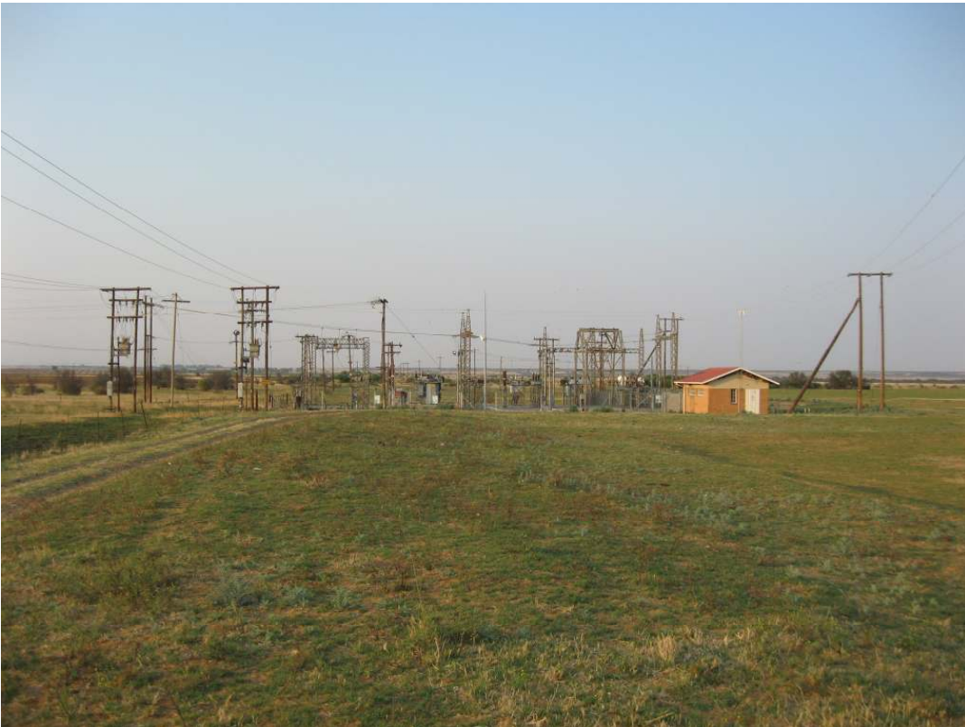
Photo 2: View of the Hoopstad substation.
