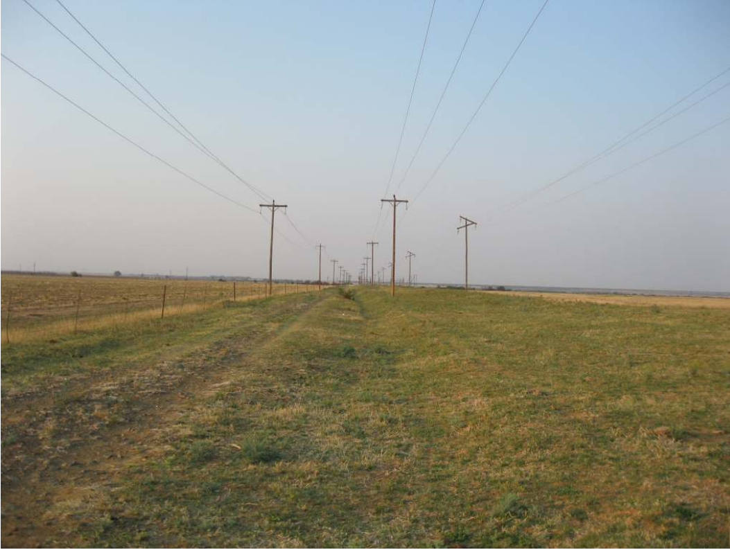
Photo 3: View of the power lines on the southern side.
