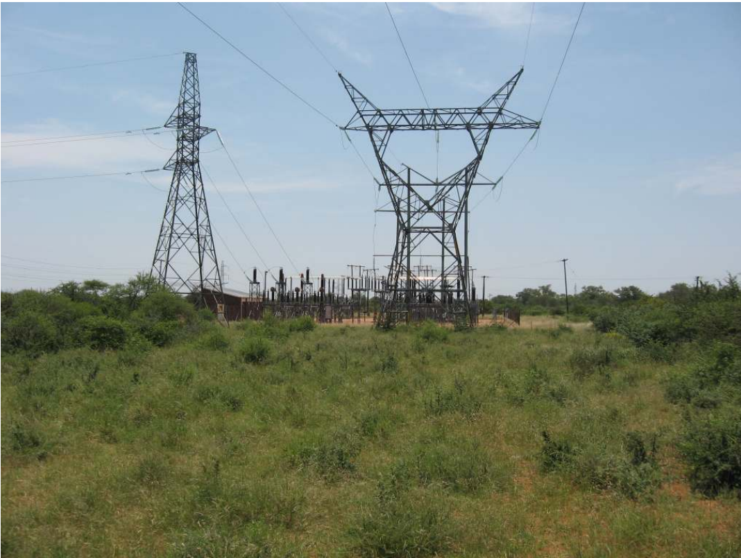
Photo 2: View of the Tom Burke Substation to the east.
