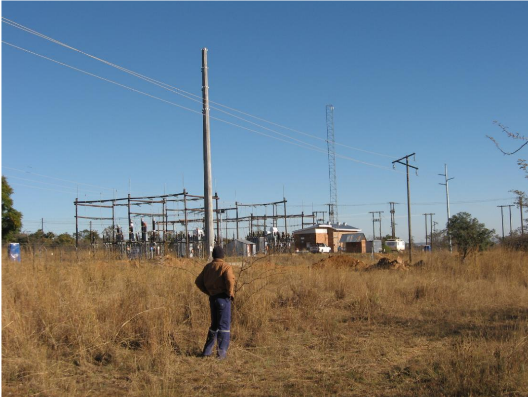
Photo 1: View of the Vaalwater Substation.
