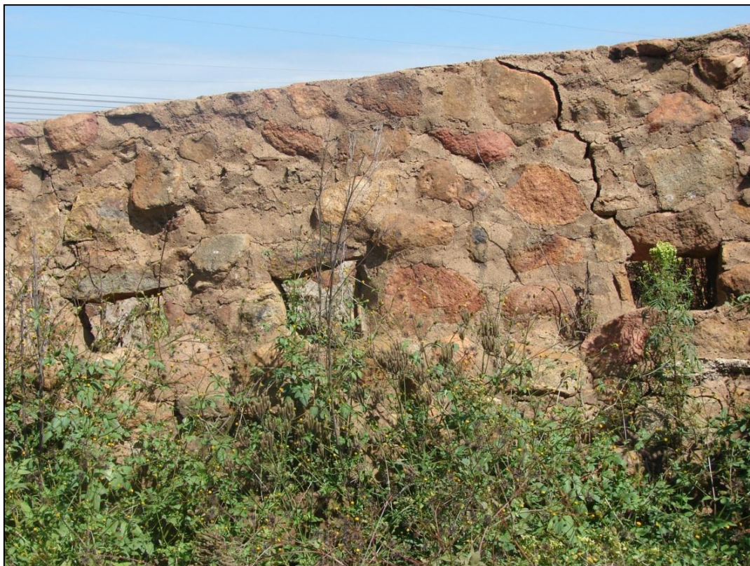
Figure 29 -Stone and mortar kraal, note small window openings on the side of the kraal wall. © Tomose @ PGS
