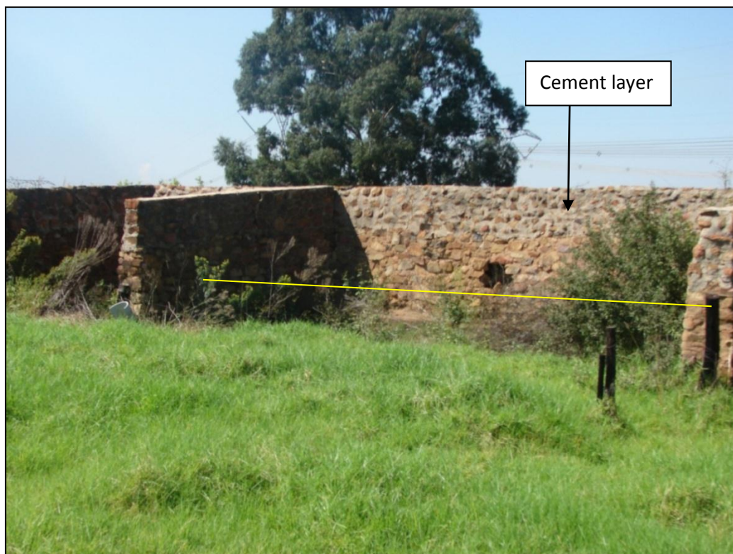
Figure 30 - Cement layer, north face of the kraal. Note the window opening; stones have fall on the window.
