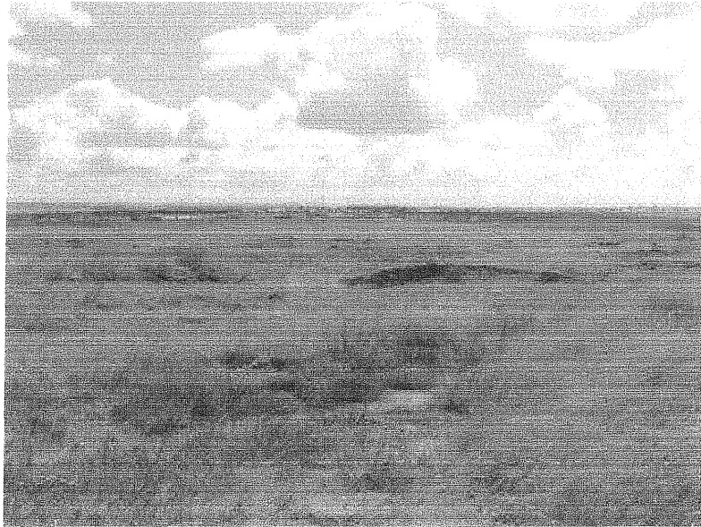
Figure 7: A closer view of the already disturbed area where services are being installed.
