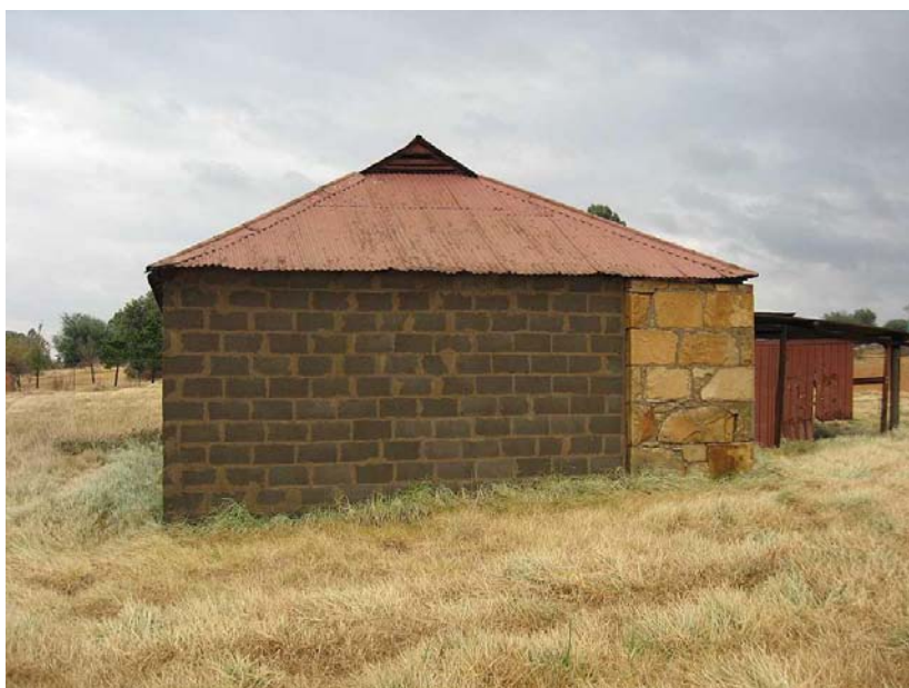
Figure 17. Site WS 4 An old sandstone built shed showing different building material
