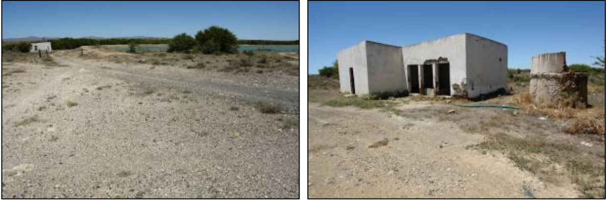
Figs 5-6. Views of the dilapidated structures.
