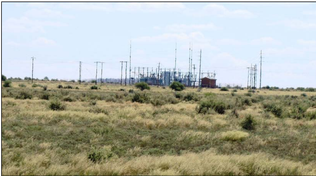
Fig.1 Osborne Sub-Station at Wicklow 218, Hopetown.
