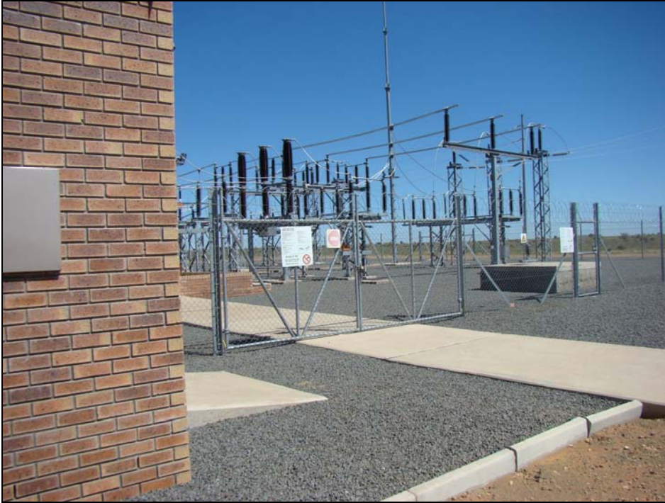
Fig.2 Osborne 132/22kV Sub-Station at Wicklow 218, Hopetown.
