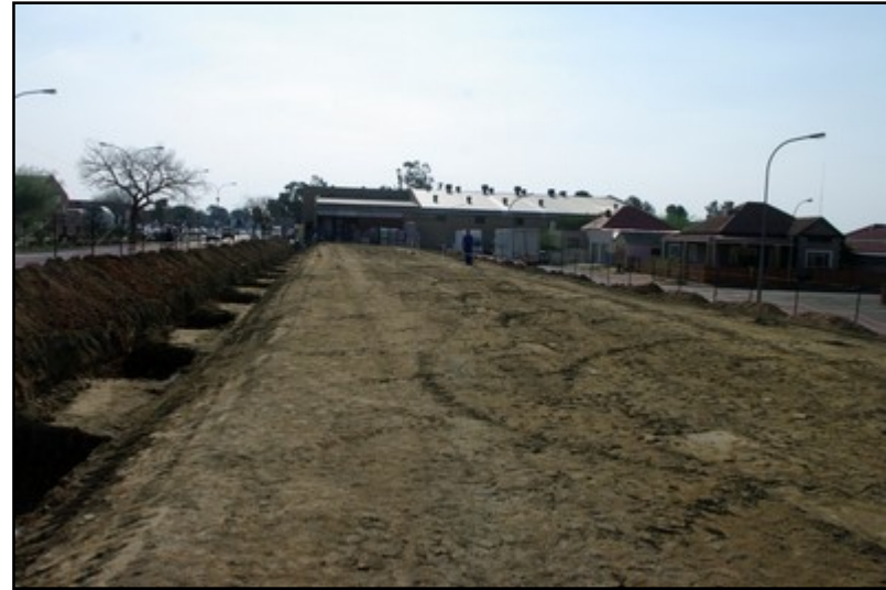
Plate 12: General site view after foundation trenching, with the Samy's wholesalers depot in the background
