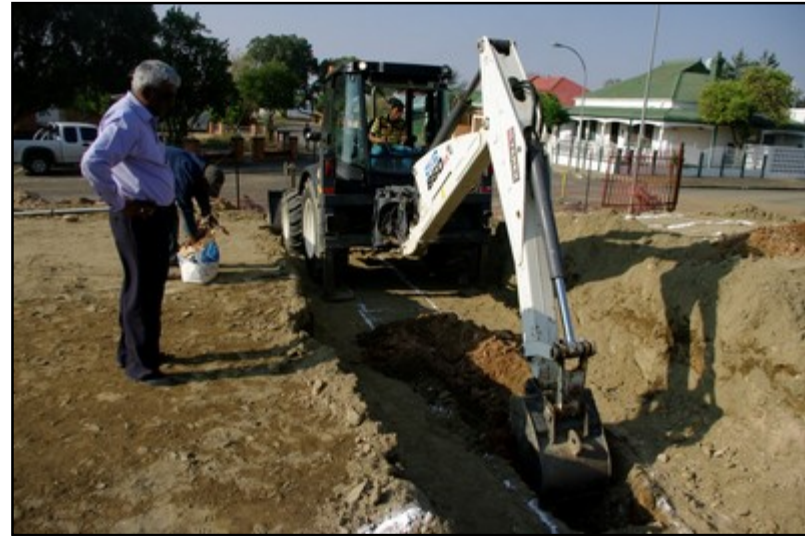
Plate 11: Excavation trenching, south-eastern corner of structure foundations, with developer Tom Pillay, P&V Pillay Family Trust
