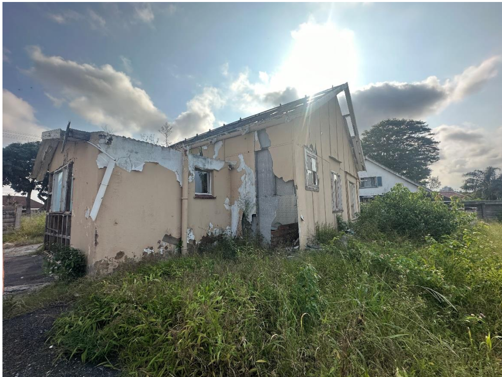
NORTH-EAST REAR ELEVATION. THE FAÇADE HAS BEEN COMPLETELY RIPPED; THE ASBESTOS HAS ALSO DETERIORATED.
