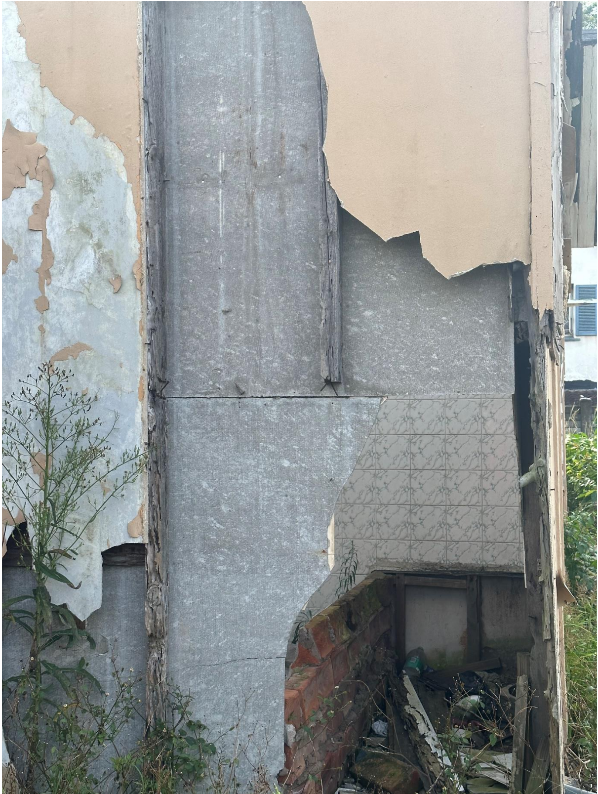
EXAMPLE OF WALL CONSTRUCTION CONSTRUCTED OUT OF ASBESTOS, WOOD FRAME PANELING AND
