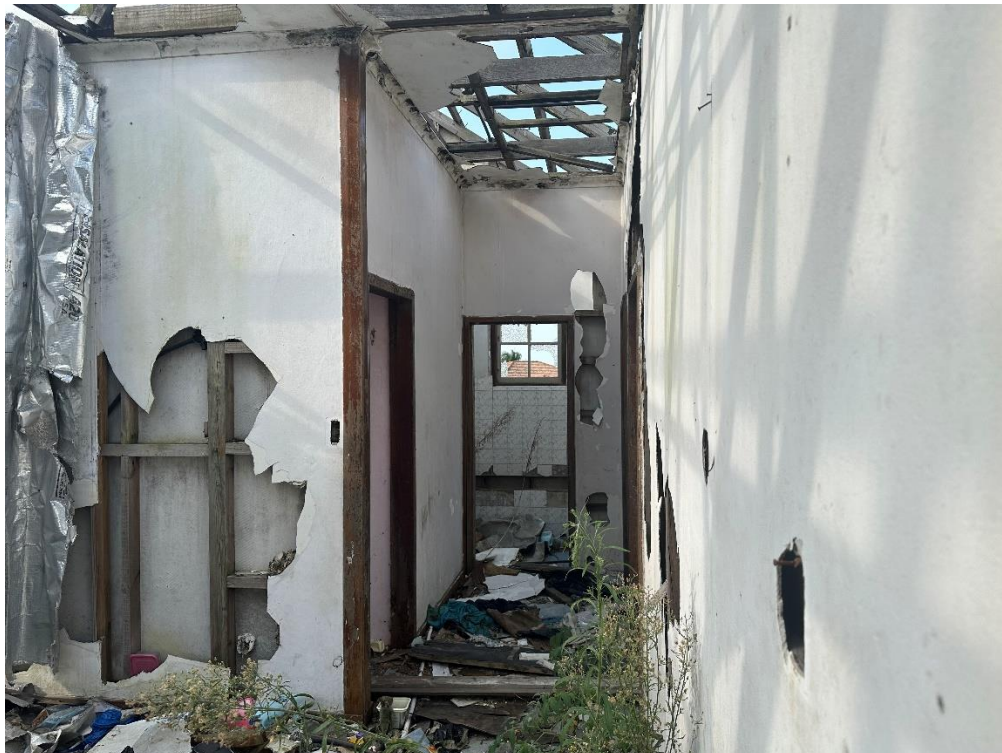
INTERIOR VIEW OF HOUSE – DAMAGED WALLS AND FLOOR, THE ROOF HAS BEEN COMPLETELY STRIPPED
