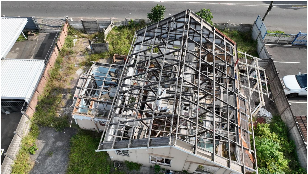
AERIAL VIEW OF DAMAGED AND STOLEN ROOF
