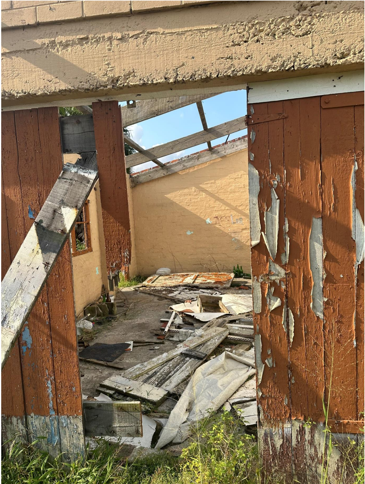
INTERIOR VIEW OF GARAGE, ONE CAN OBSERVE THE STRUCTURE IS COMPLETELY STRIPPED/
