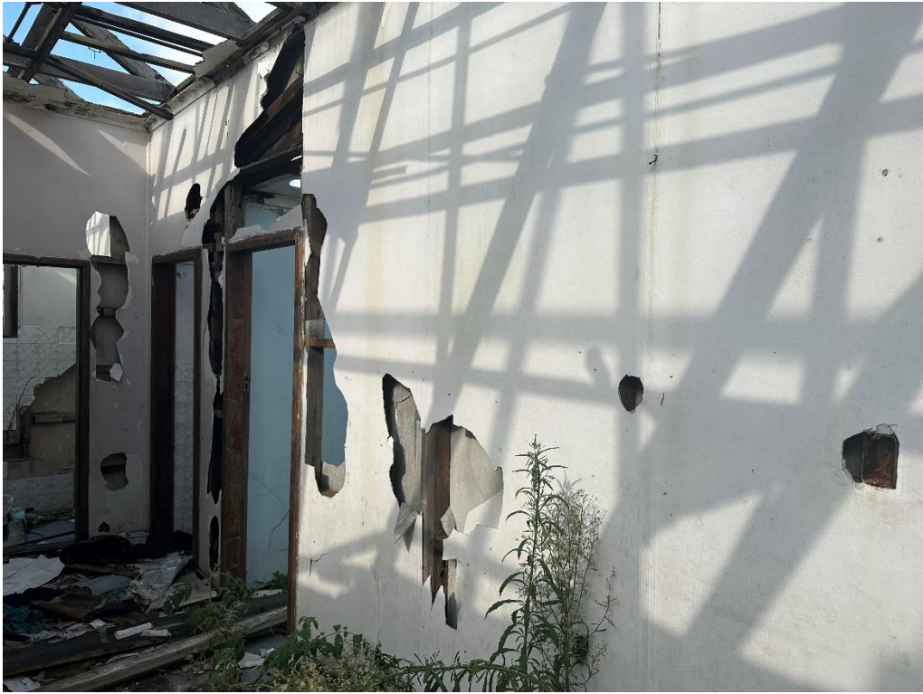
INTERIOR VIEW OF MAIN HOUSE, SHOWING EXTENSIVE DAMAGE
