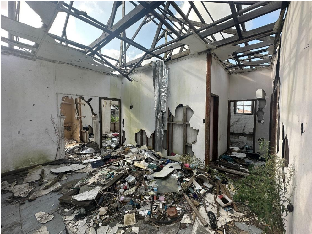
INTERIOR VIEW OF HOUSE – DAMAGED WALLS AND FLOOR, THE ROOF HAS BEEN COMPLETELY STRIPPED
