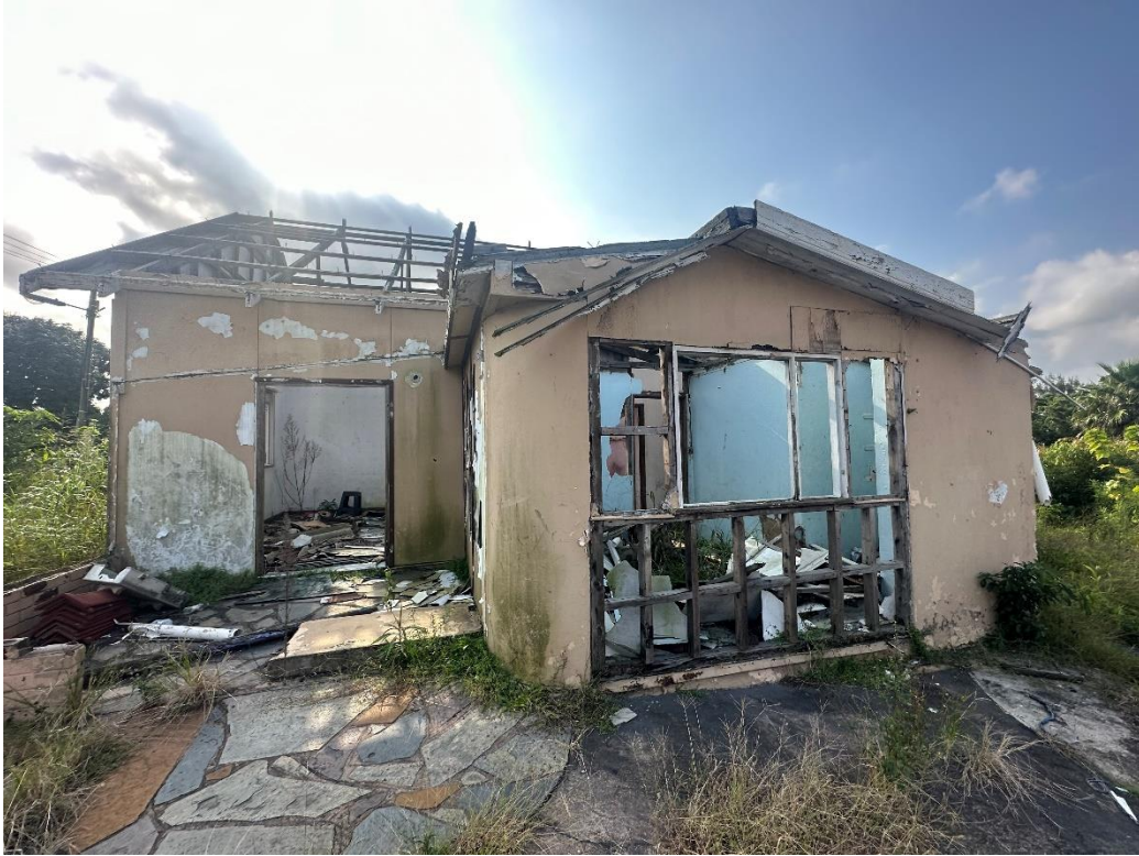
NORTH-WEST ELEVATION, ENTRANCE VIEW. AGAIN ONE CAN OBSERVE THAT THE STRUCTURE HAS DETERIORATED AND THE WOOD THAT HAS ROTTEN
