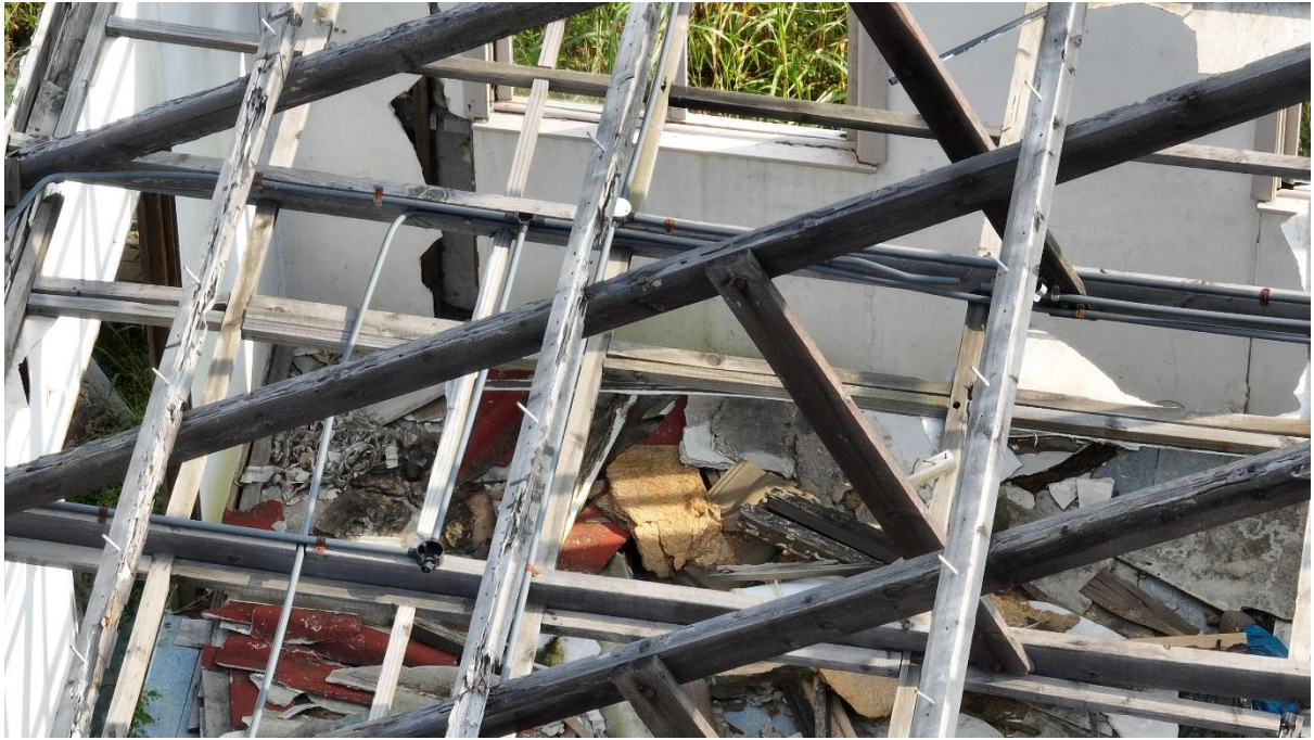
AERIAL IMAGE ZOOMED IN SHOWING DAMAGED ROOF
