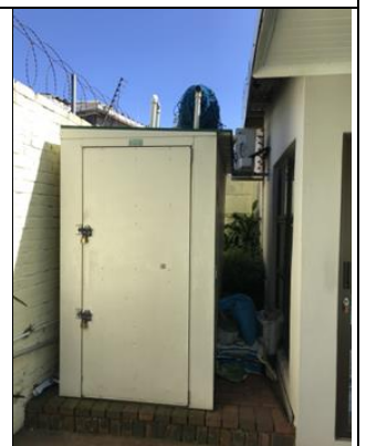
Generator - Outbuilding West End
