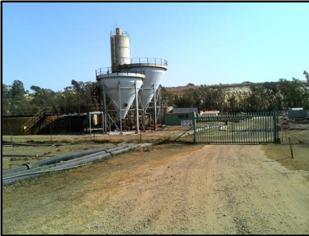
Figure 6: Existing treatment works.
