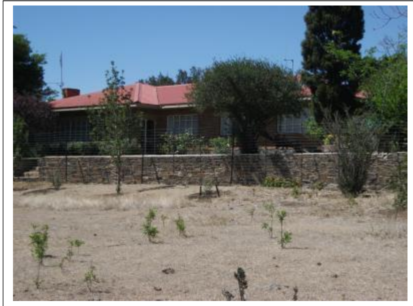
Figure 10- The main residence (FC01.1) in FCO1 comprises a multi-room dwelling which was built with clay bricks and fitted with a pitched corrugated iron roof and steel window frames (above).
