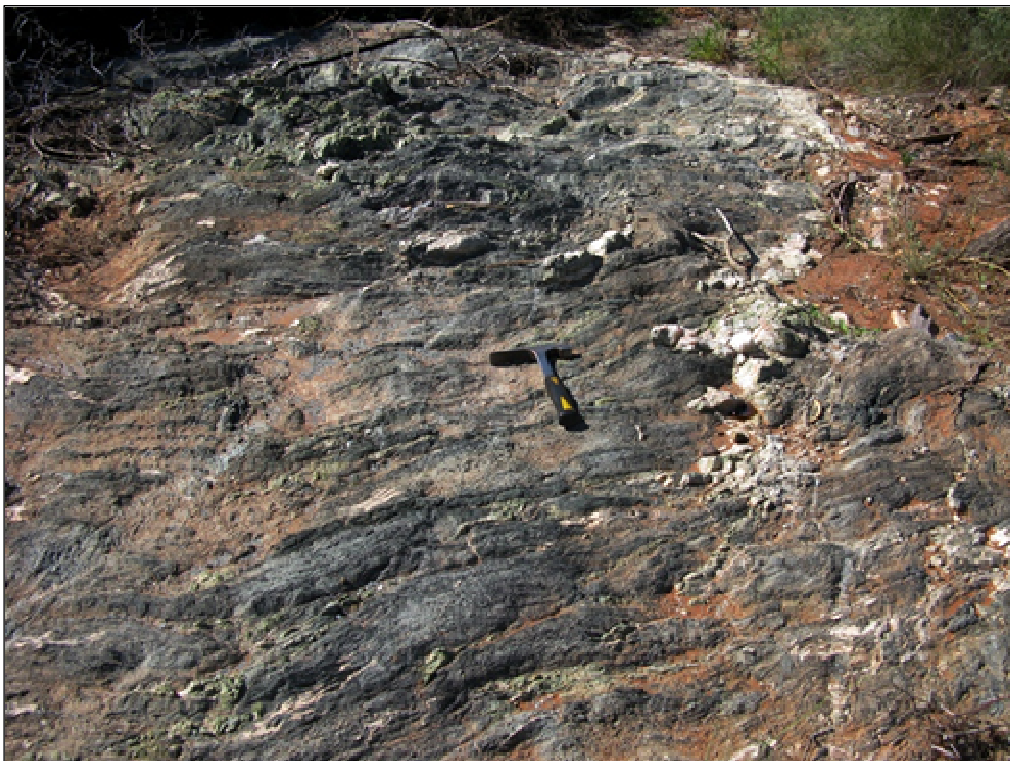
Fig. 4. Bedrock exposure adjacent to footings of Bridge 3 showing highly foliated schists of the Leerkrans Formation (Wilgenhoutsdrif Group) that are cross-cut by quartz veins (Hammer = 32 cm).
